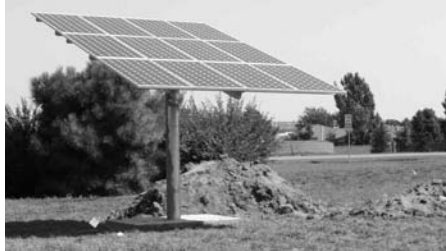
PVREA cut the ribbon on its solar demonstration project in 2007.
