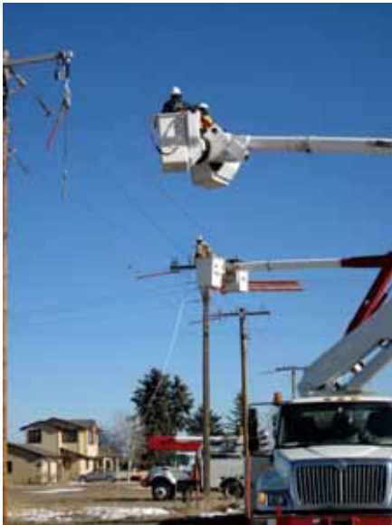
Two line crews work to replace power lines with new, larger conductor on Vine Street near Fort Collins in January 2011
